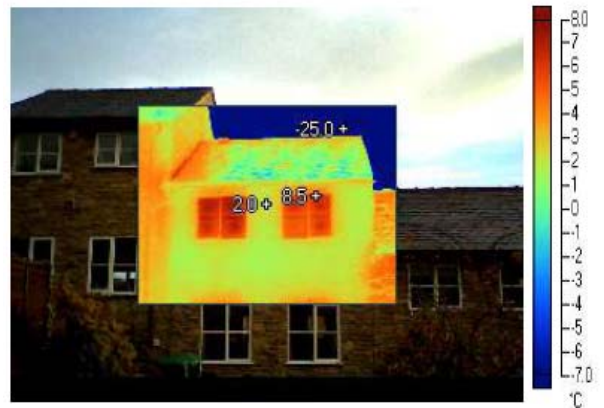
Photos: Cavity insulation – Nov 2009 (notice the colour change in the walls compared with next door)
