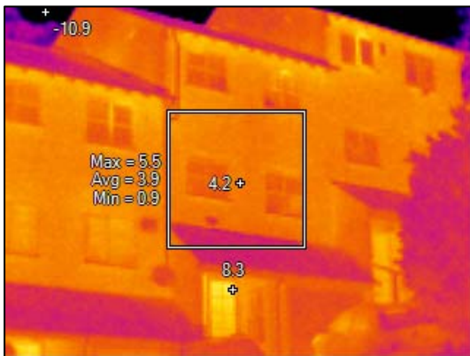
Photos: No cavity insulation – Nov 2007
