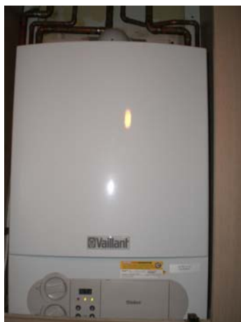
Photos: A+ rated boiler Dec 09 (only 1 month of savings realised)
